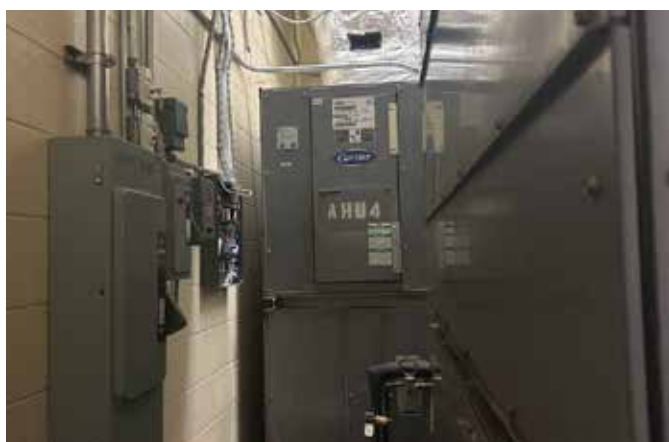
Air Handling Unit and Power Supply
