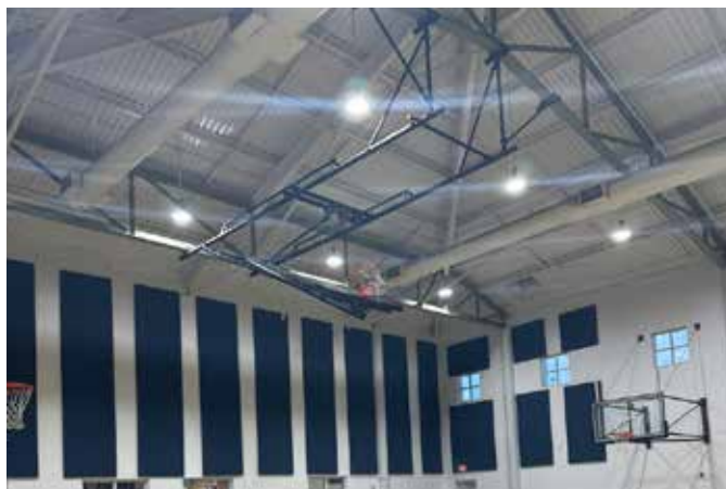
Gymnasium Exposed Structural and HVAC System
