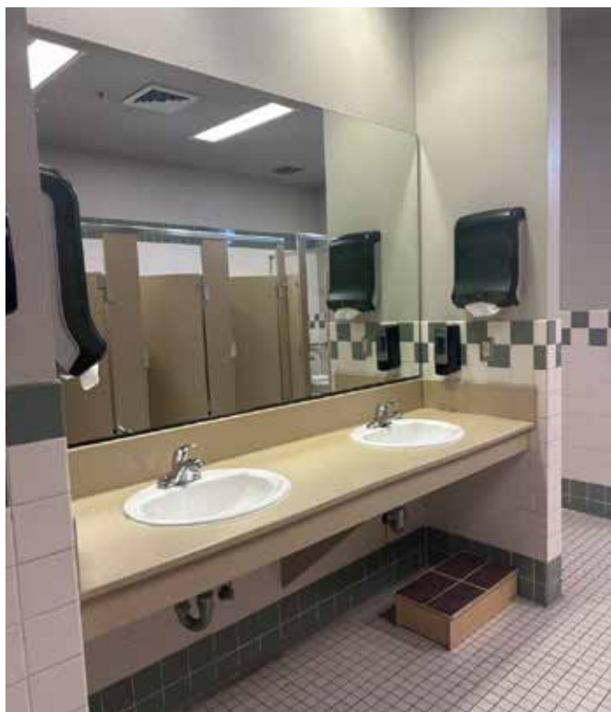
Counter with Exposed Pipes
