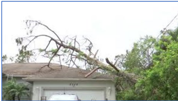
Figure 5. Tree from undeveloped lot that fell on house.
