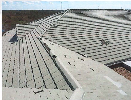
Observation - Tiles It appears a large amount of tiles have been broken throughout the roof system at this time, These items should be re set to ensure the system will continue to stay water tight.
