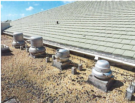
Observation - Mechanical equipment Mechanical equipment still appears to be attached and is properly secured to the curb at this time.
