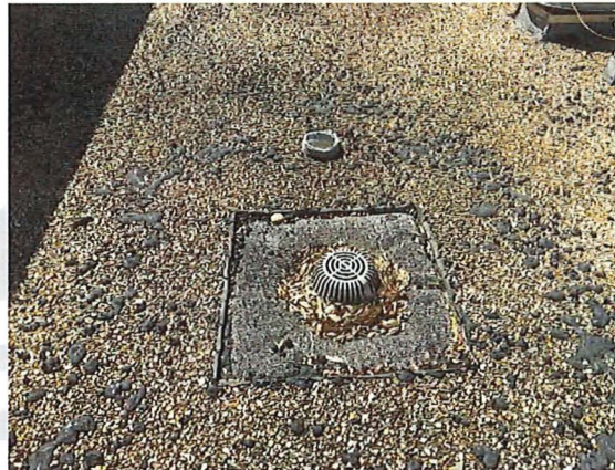
Observation - Drain's Roof drain's appear to be performing well but are currently surrounded by leaf debris.
