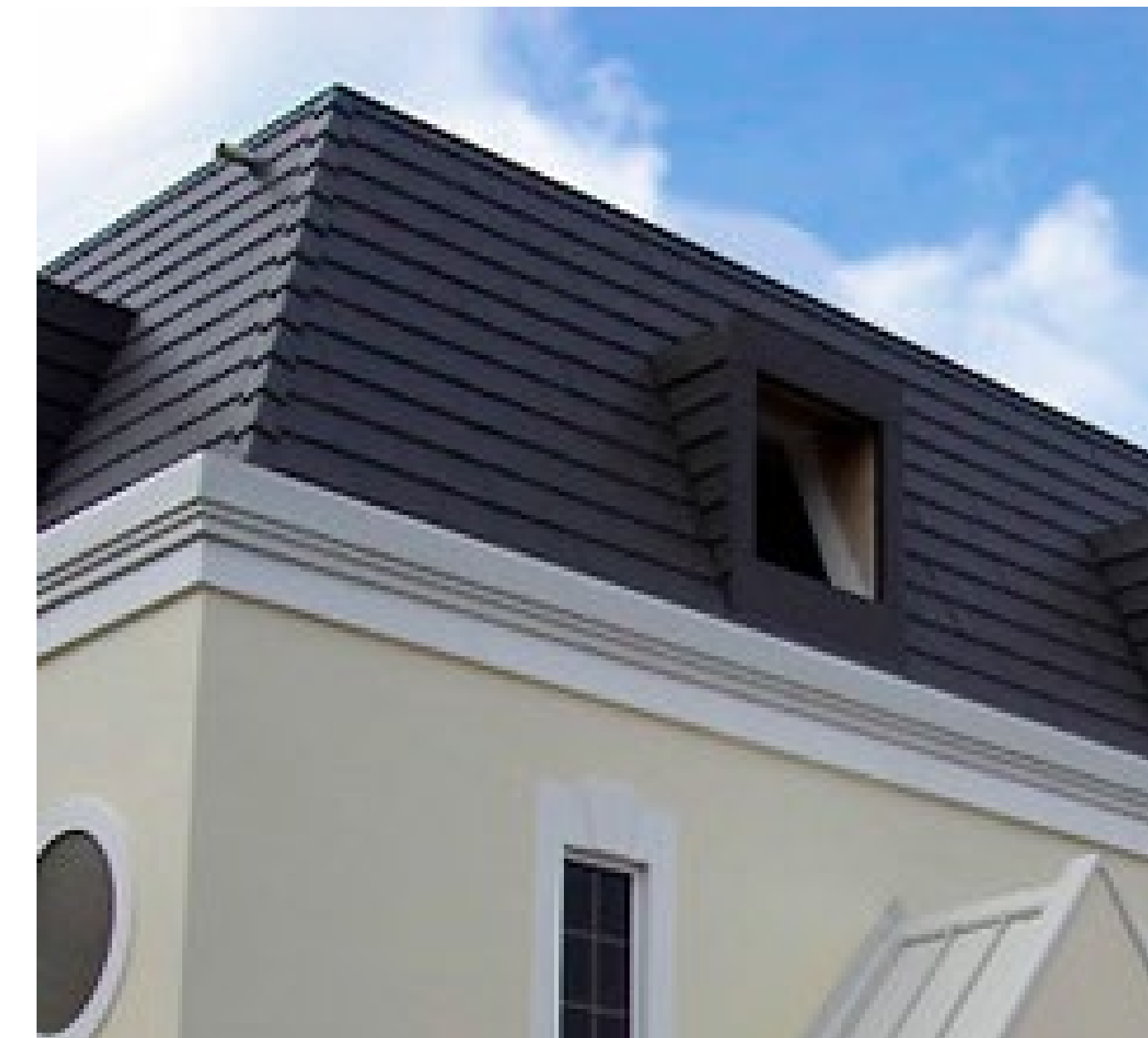
FIGURE 11.5.1.B Non-residential and multi-family buildings may have flat roofs but should use a mansard wall to screen edges and mechanical units.
