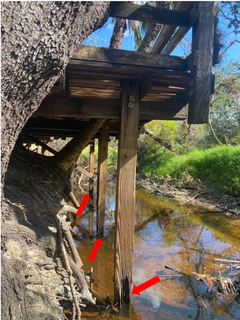
Photograph 4 – Damaged Piles In Observation Deck
