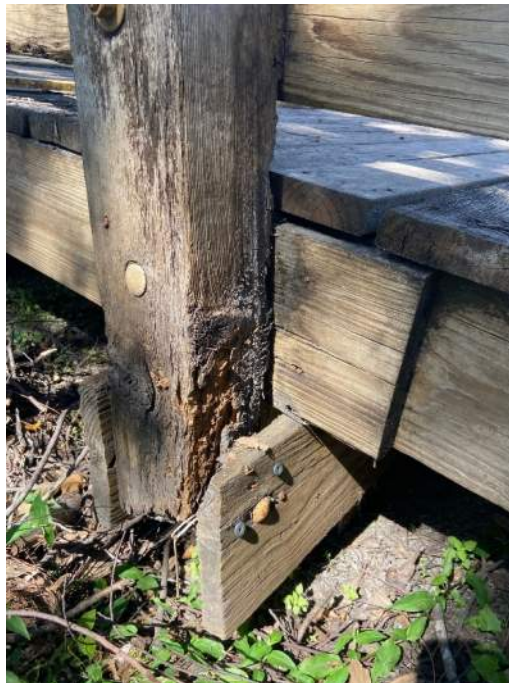
Photograph #5B: Damaged Girder and Handrail Post
