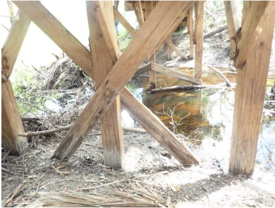
Photograph #3: Damaged Brace
