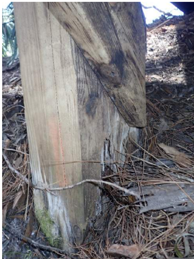
Photograph 2 – Closeup Of Damaged Piles In Equestrian Bridge
