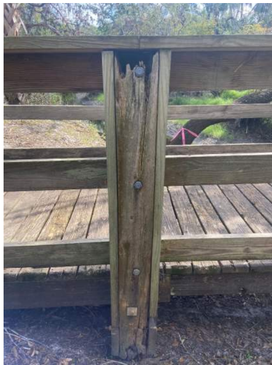
Photograph #16: Damaged Post
