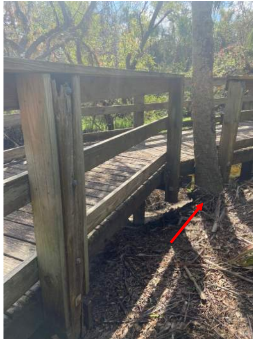
Photograph #15: Tree Very Close by to Deck
