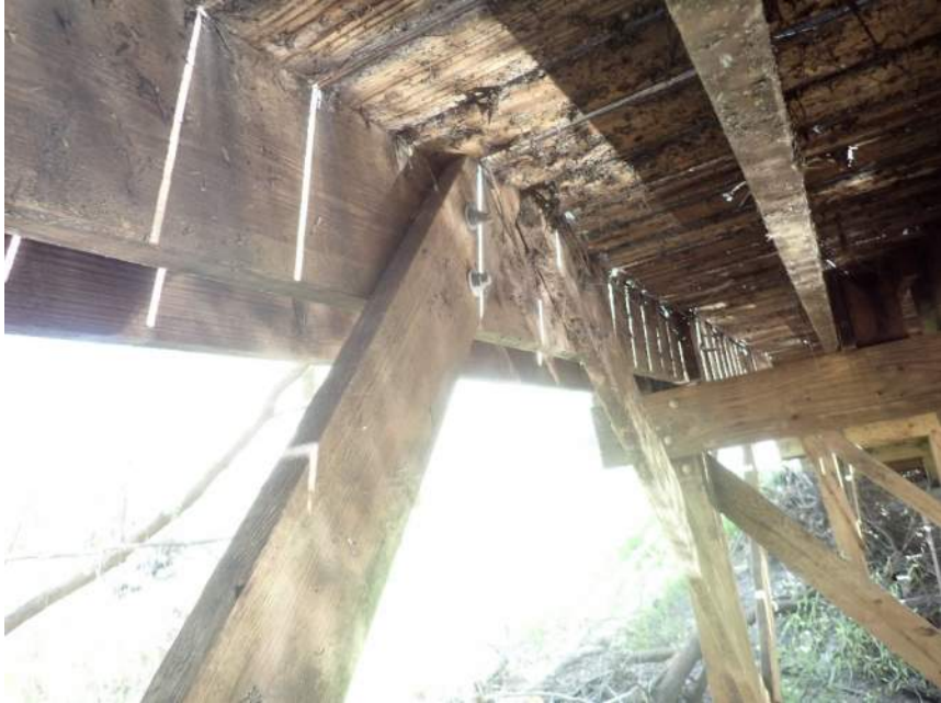
Photograph #11: Debris Underside the Deck
