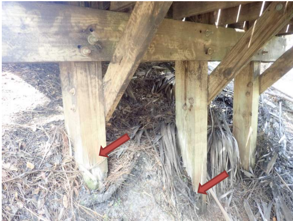
Photograph 1 – Damaged Piles In Equestrian Bridge
