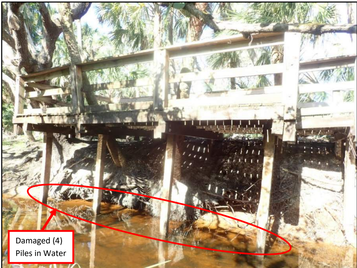
Photograph 2 – Observation Deck with Damages
