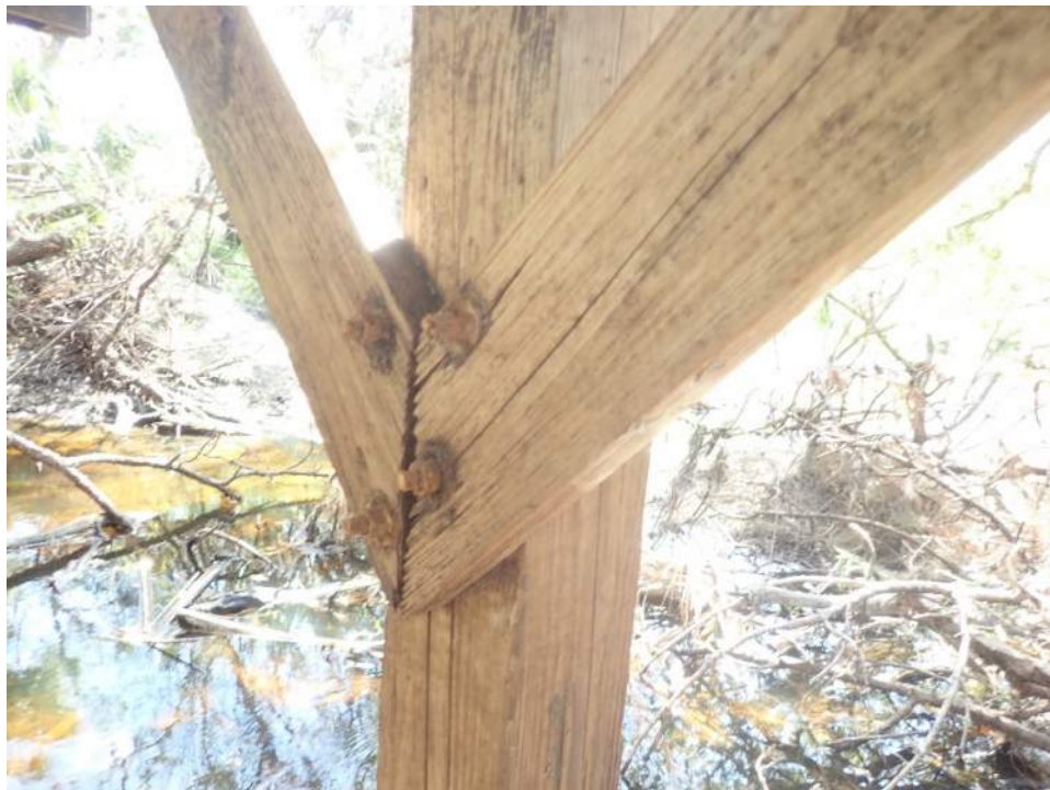
Photograph #4: Corroded Bolts
