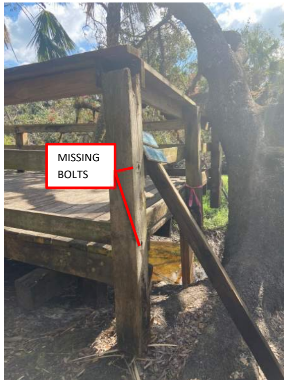
Photograph #17: Damaged Post
