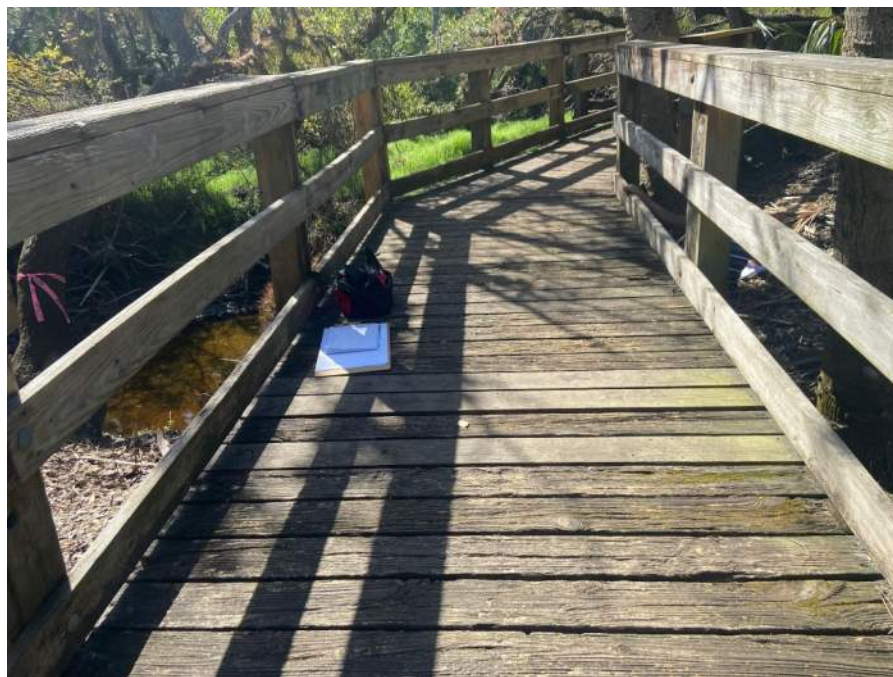
Photograph #18: Damaged Deck
