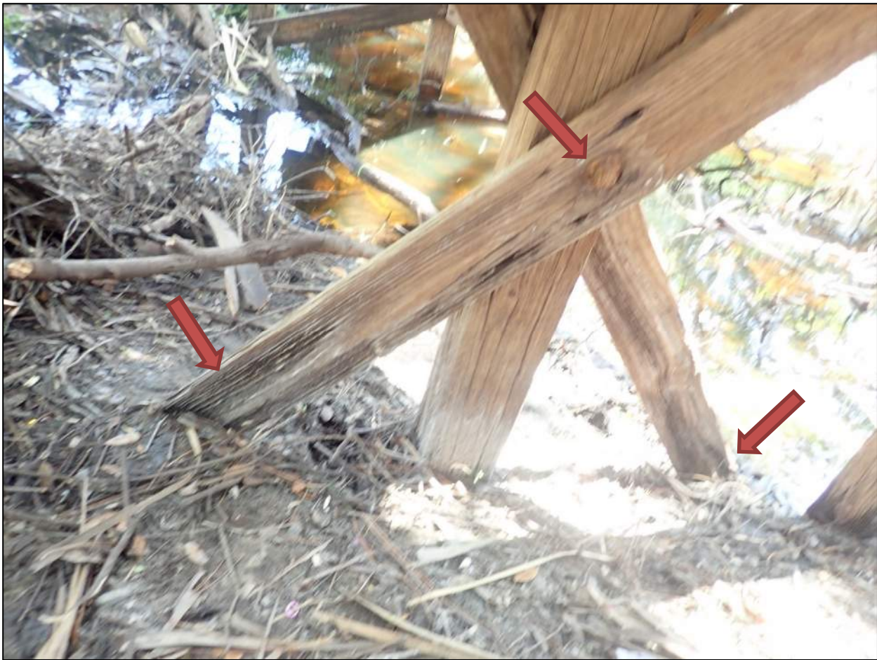
Photograph 3 – Example of Damaged Bracing In Equestrian Bridge
