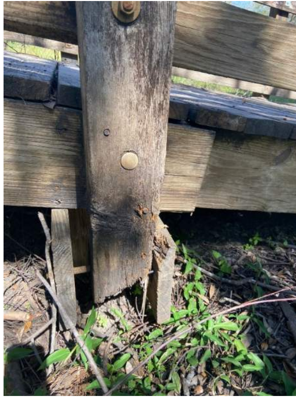
Photograph #5A: Damaged Girder and Handrail Post
