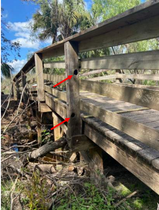
Photograph #8: Bird Damage at Post
