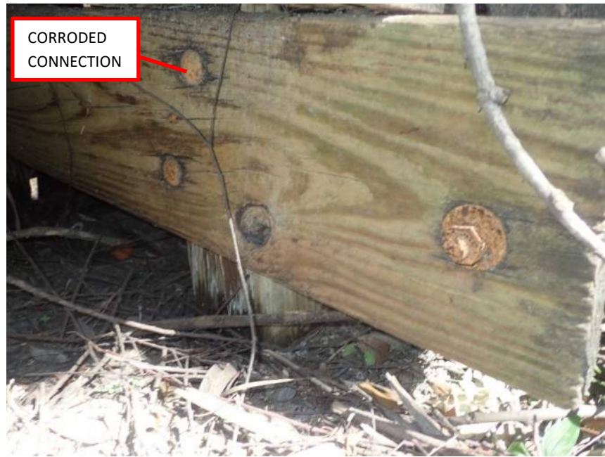
Photograph #5C: Corroded Girder to Beam Connection
