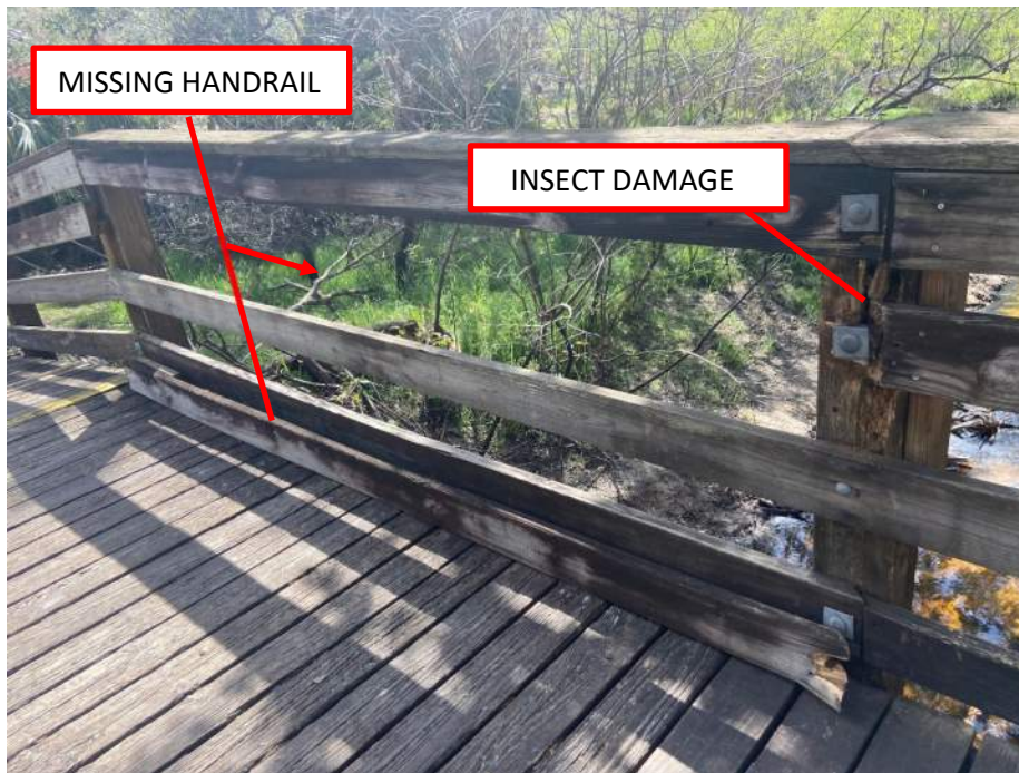
Photograph #9: Beam Missing on Handrail
