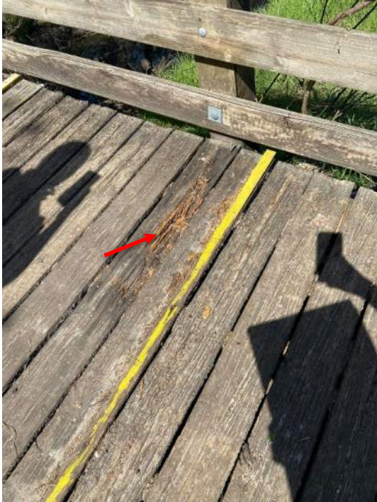
Photograph #7: Rotten Deck
