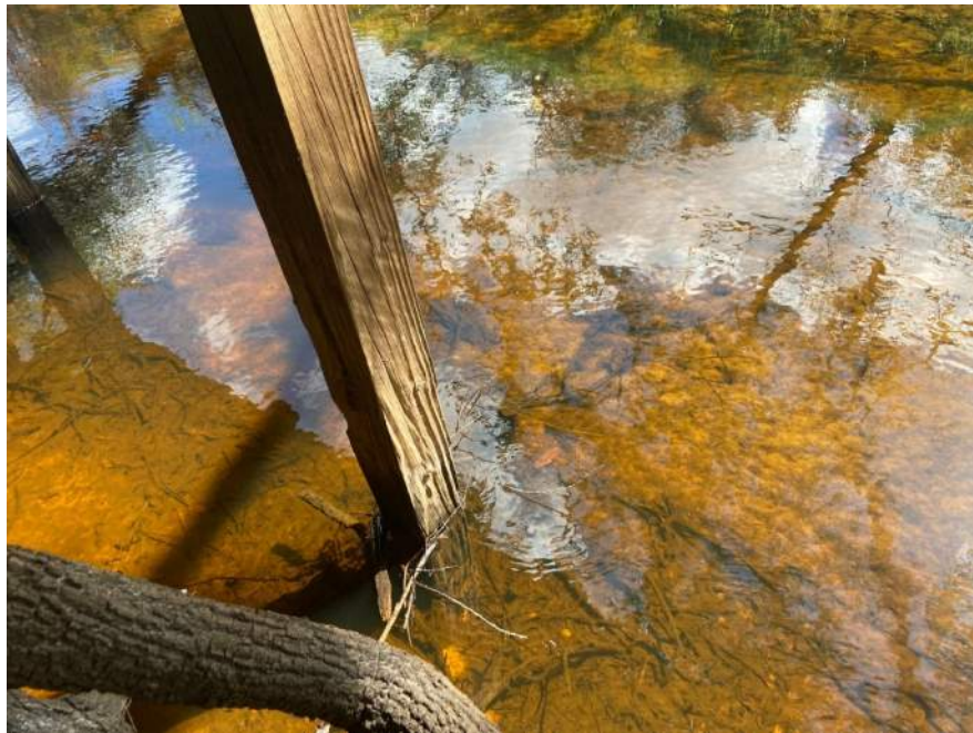
Photograph #13: Damaged Pile
