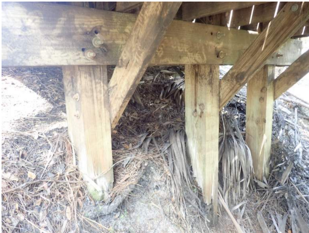
Photograph #2: Damaged Piles
