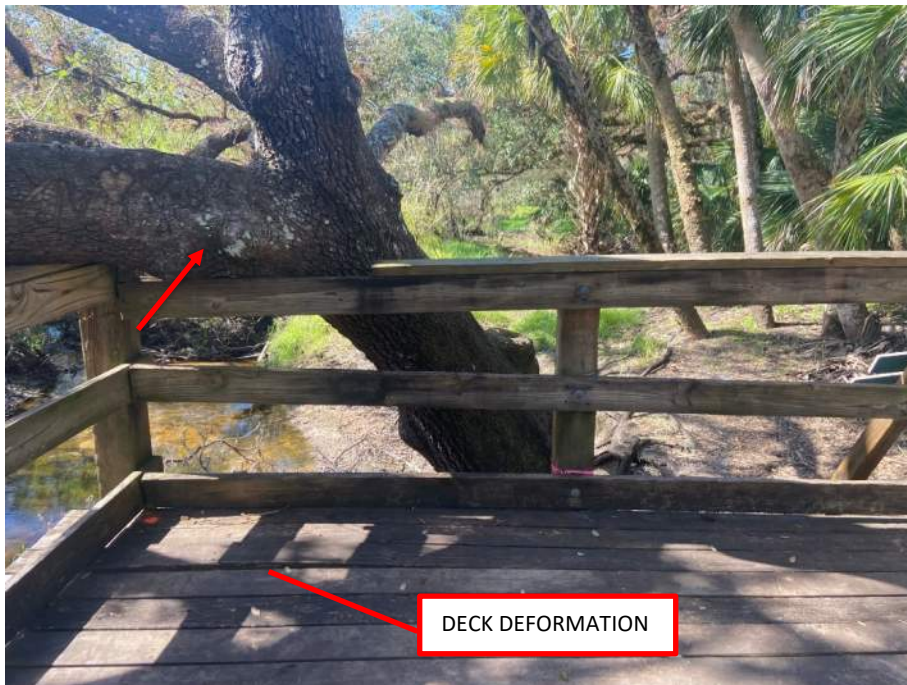
Photograph #14: Tree Branch Resting on Handrail
