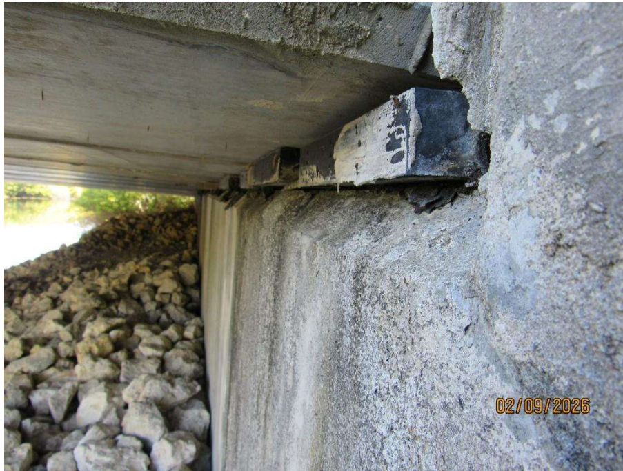
Photo 3: Abutment 1 bearings walking out.
