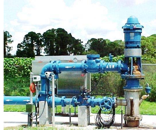
Aquifer Storage & Recovery Piping
