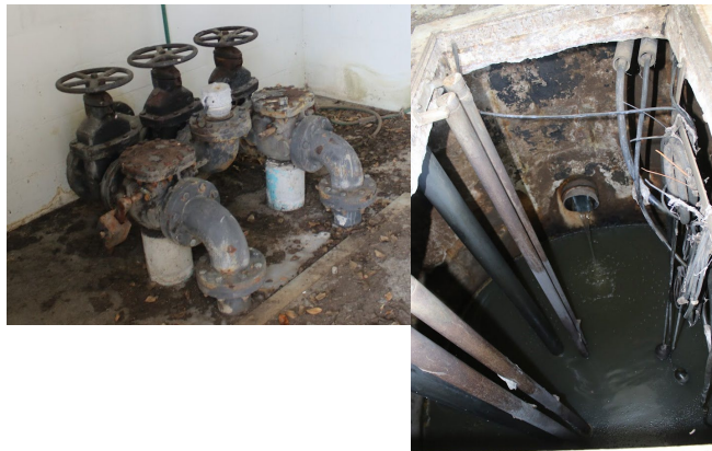
Sample Pictures of Aging Utility Infrastructure in North Port
