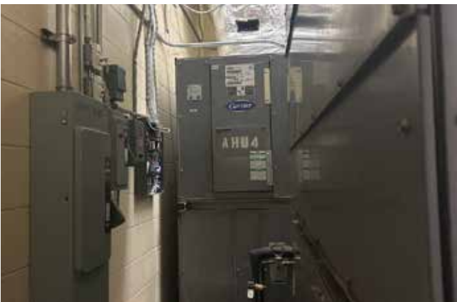
Air Handling Unit and Power Supply
