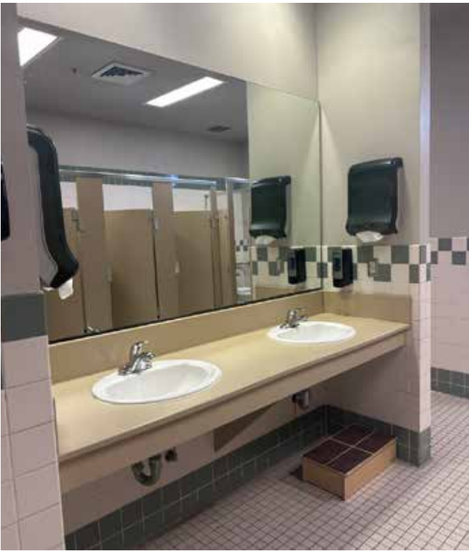
Counter with Exposed Pipes
