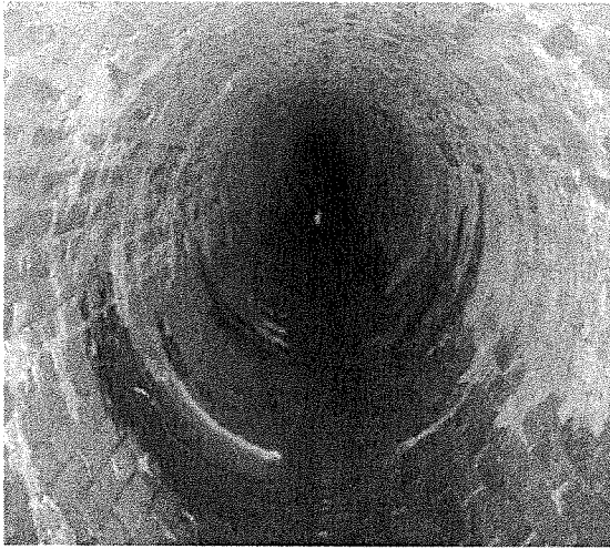
*Locate Infiltration or Defect
