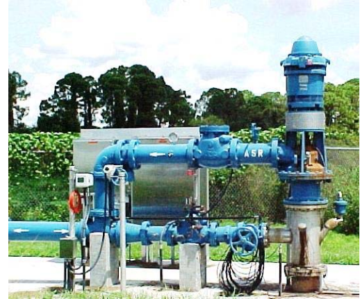
Aquifer Storage & Recovery Piping
