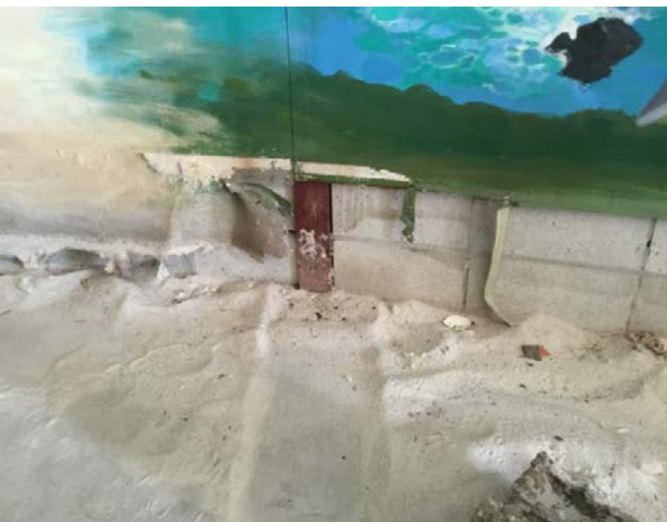
Picture 17 Building 3 - Cyclorama Steel Column in Wall
